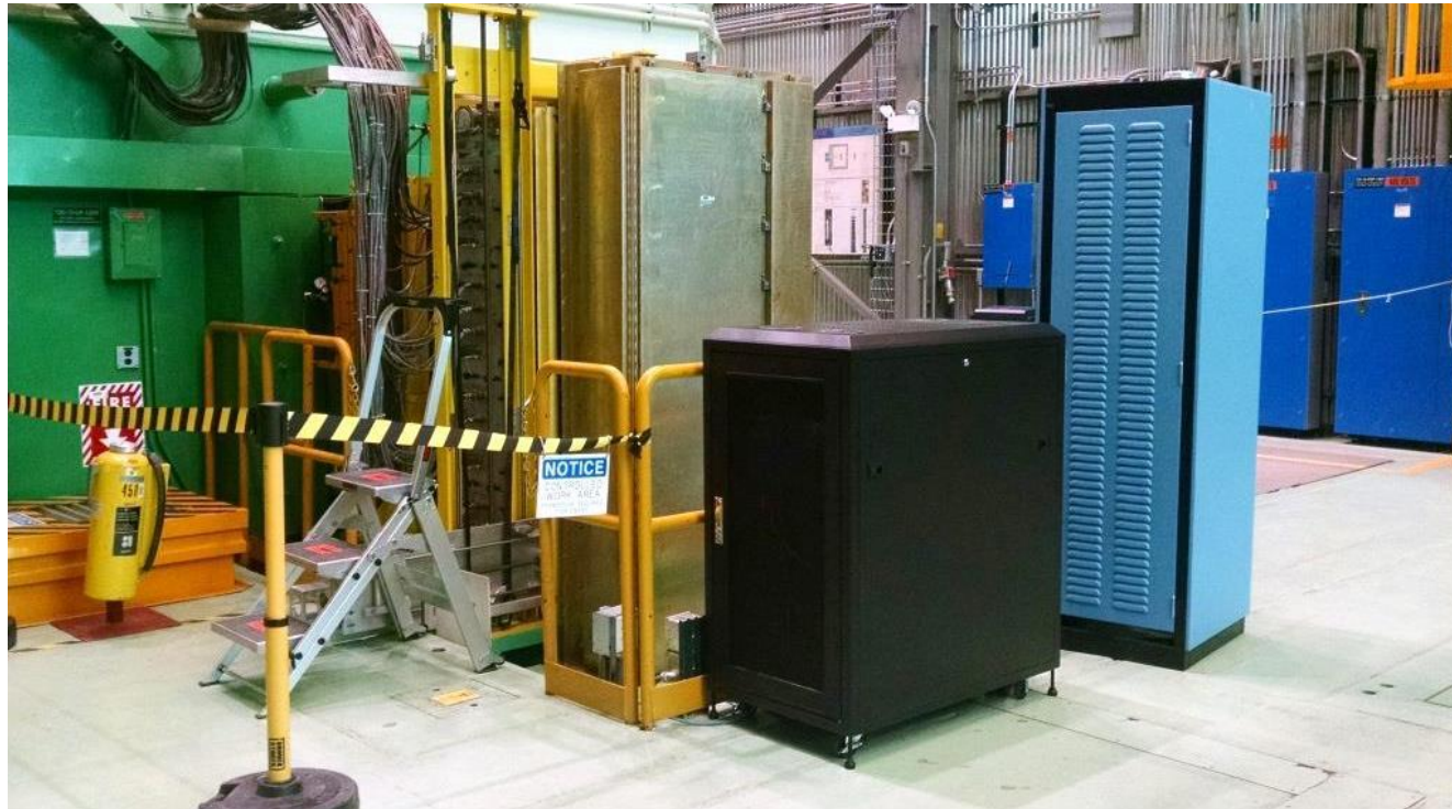
View of the Hodoscope system including cabinets
