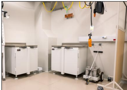
Lead-shielded cabinets, barriers, and cart
