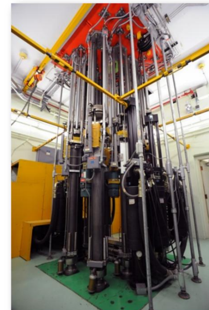
TREAT subpile room
